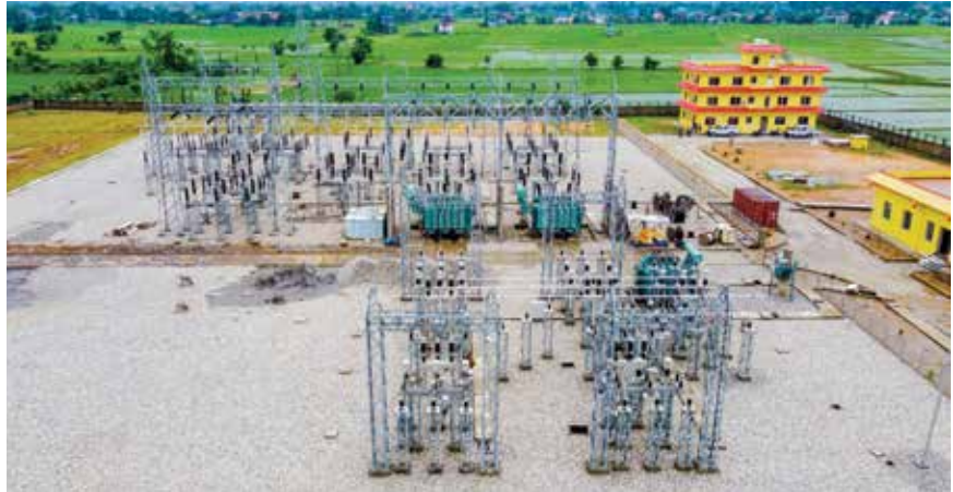
▲ Purbi Chitwan 132-11kV Substation constructed by NHE
